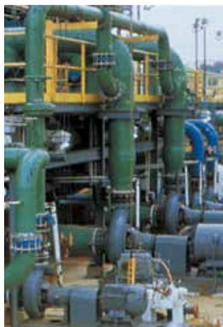
3175's on process service such as multi-effect evaporators.
