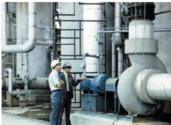
A 3175 installed in a major chemical plant.
