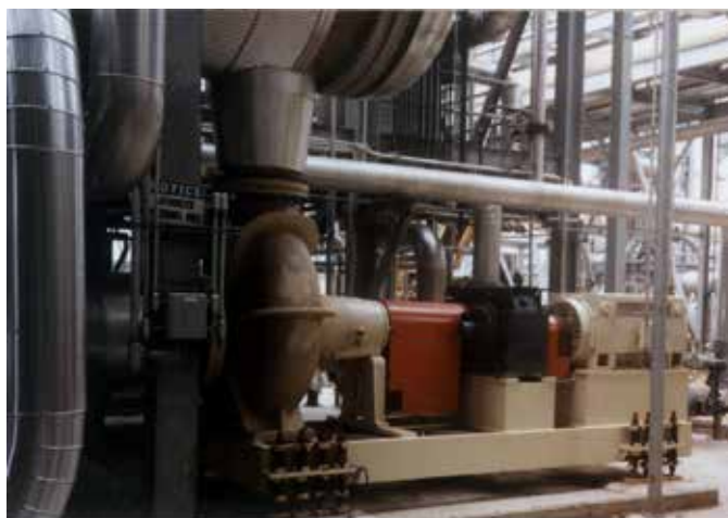
Black liquor circulation pump (3175 XL) on spring-loaded baseplate.
